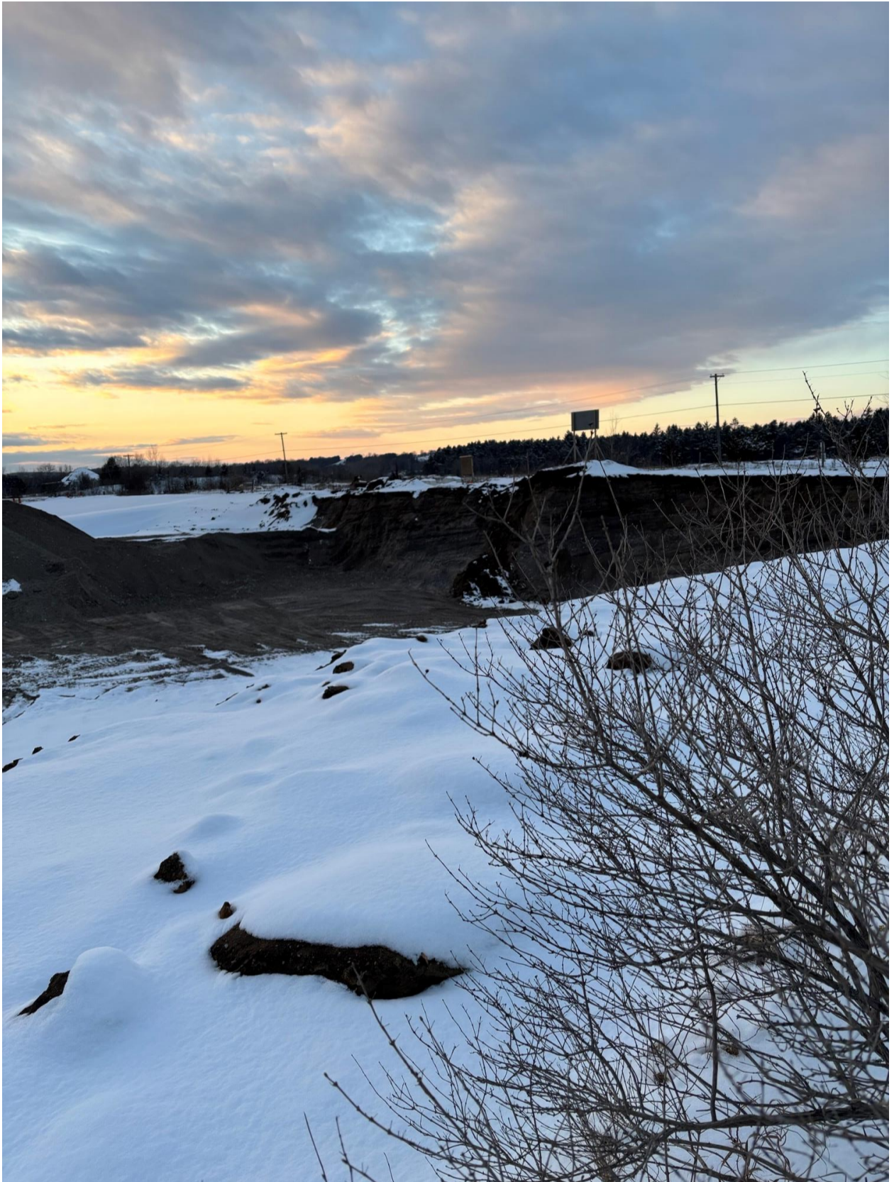
This picture Taken January 27 th 2025 shows the depth of the excavation of the Rural Residential Lots on Little Lake Rd and Trent Vally Road. The depth of the excavation is approximately 40 ft. The sign seen at the top of the picture is at road level.
