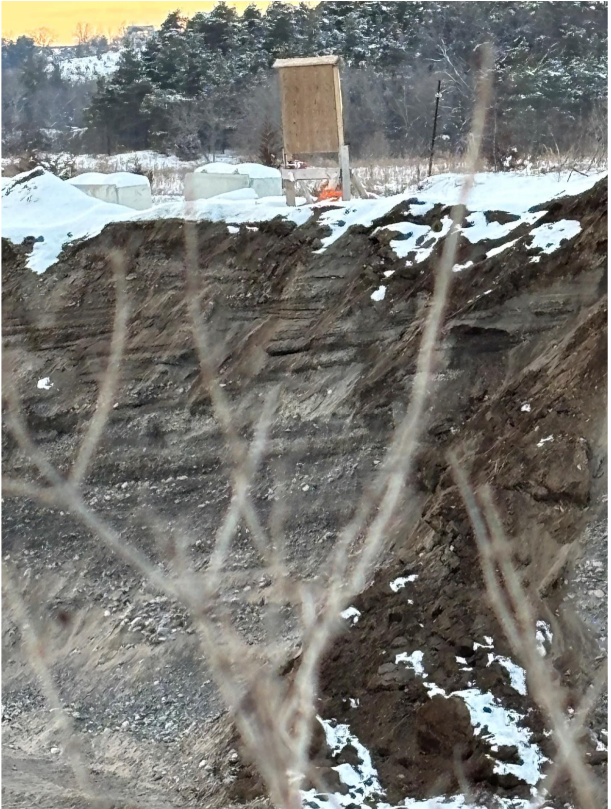
This picture Taken January 27 th 2025 shows the depth of the excavation of the Rural Residential Lots on Little Lake Rd and Trent Vally Road. The depth of the excavation is approximately 40 ft. The sign seen at the top of the picture is at road level.
