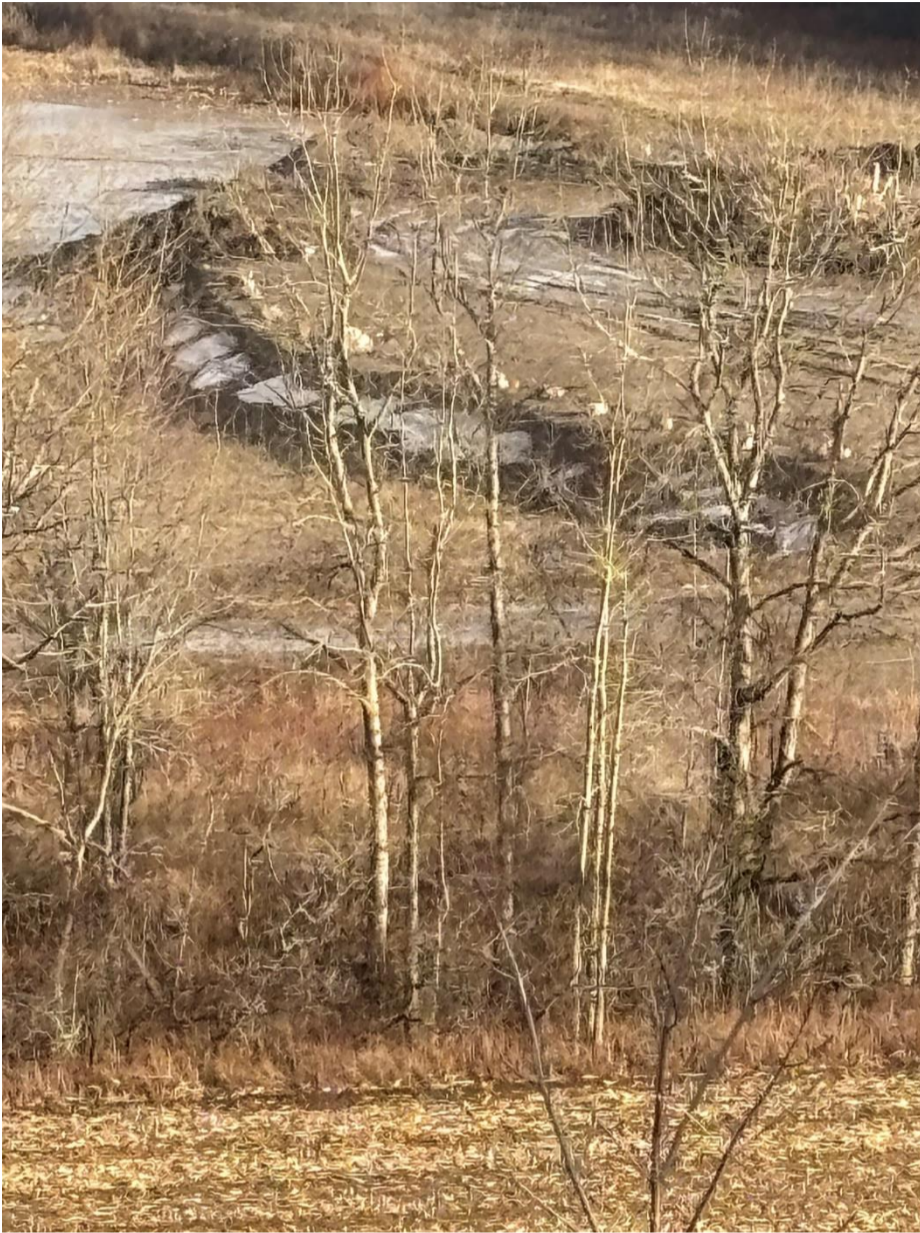
This picture was taken December 16, 2024 and shows the dumping of fill into the subject area next to the Environmental area. A closer look at the built-up area indicates the area was reinforced with materials to stabilize the foundation. Dump trucks and Quarry Trucks full of fill from two lots recently rezoned as RR and located on Little Lake Rd were brought in, piled and deposited into this area.
